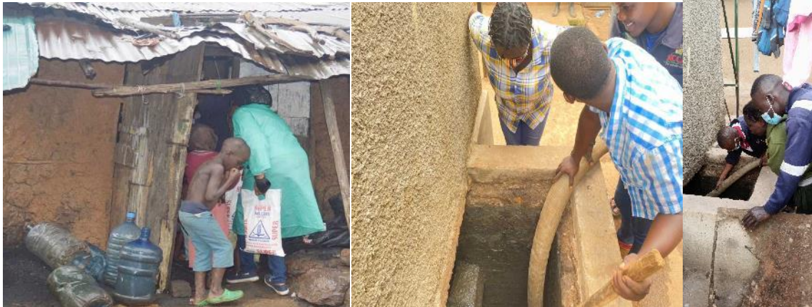
Home visits, food items distribution and emptying of pit latrines and cleaning of trenches
